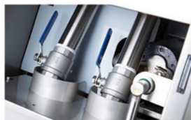
Built-in oil system
